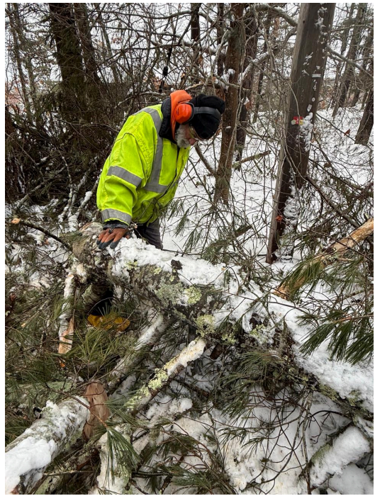
Ted inspects the tangle of tree limbs for safe removal from the damaged lines.
