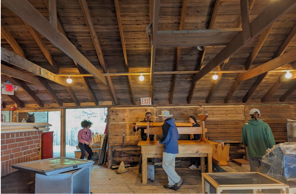
Taking the Dining Hall apart, to put it back together. Work Weekend I 2024. Photo Credit: Beth Reagan
