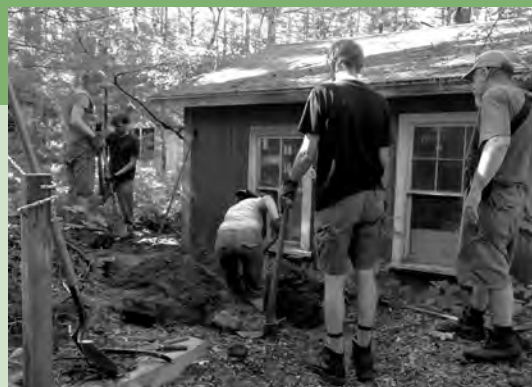
Work Weekend volunteers help Tony Baker dig a trench for the new waterline from "Amsterdam" to Hit & Miss.
